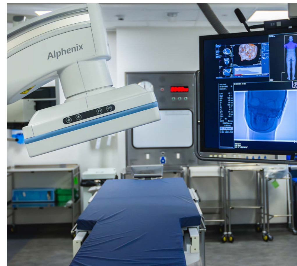
Alphenix Sky + installed at the Forth Valley Royal Hospital, Larbert, Scotland.
