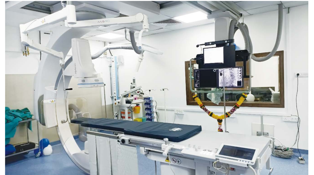
Installation at Medcover Group Hospitals India at Pune
